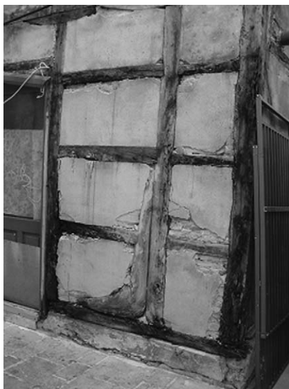
Fig. 16. Typical damage of timber framed wall.
