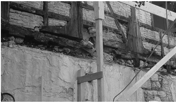
Fig. 20. Advanced decay of timber elements along the perimeter of stone masonry.
