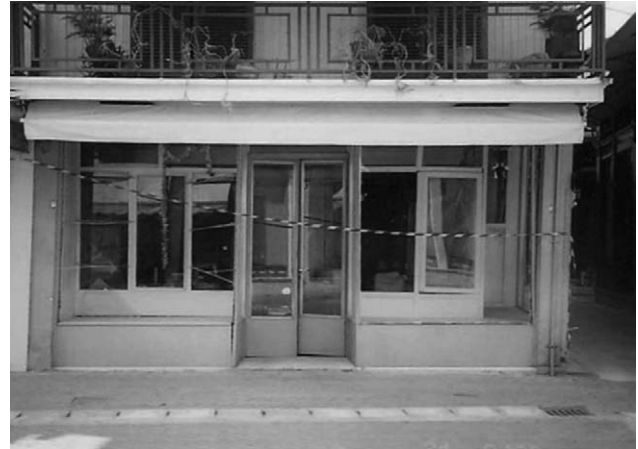
Fig. 11. Permanent interstorey drift in the ground floor.
